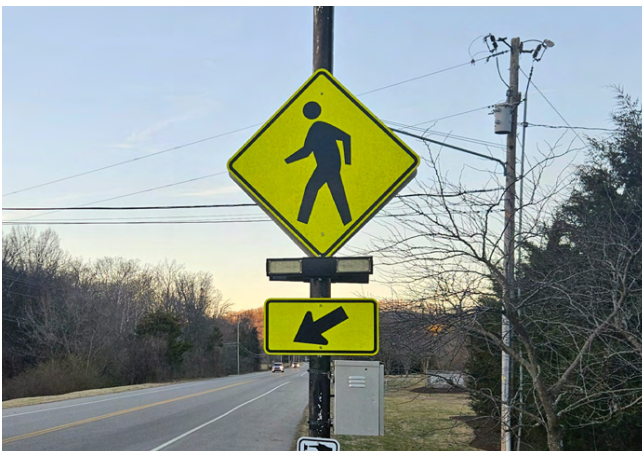
Figure 20. Rectangular Rapid Flashing Beacon (RRFB)
