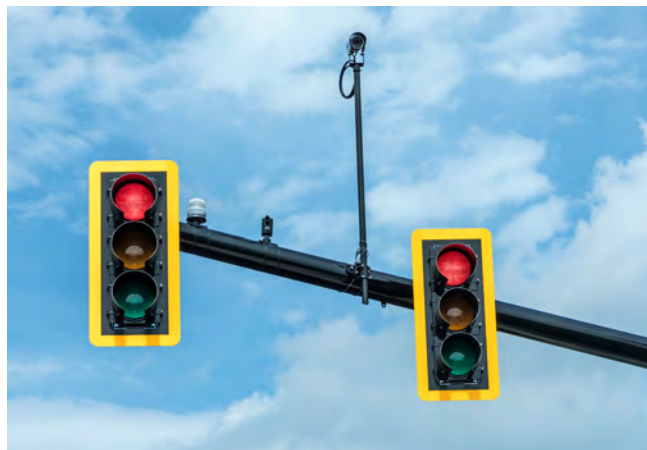
Figure 16. Signal Head on Mast Arm
